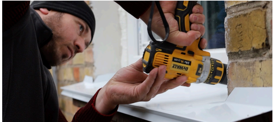
Ukrainians repair their war-damaged houses with cash assistance, helping them to return home and prepare for winter. Photo courtesy of Caritas Ukraine staff
