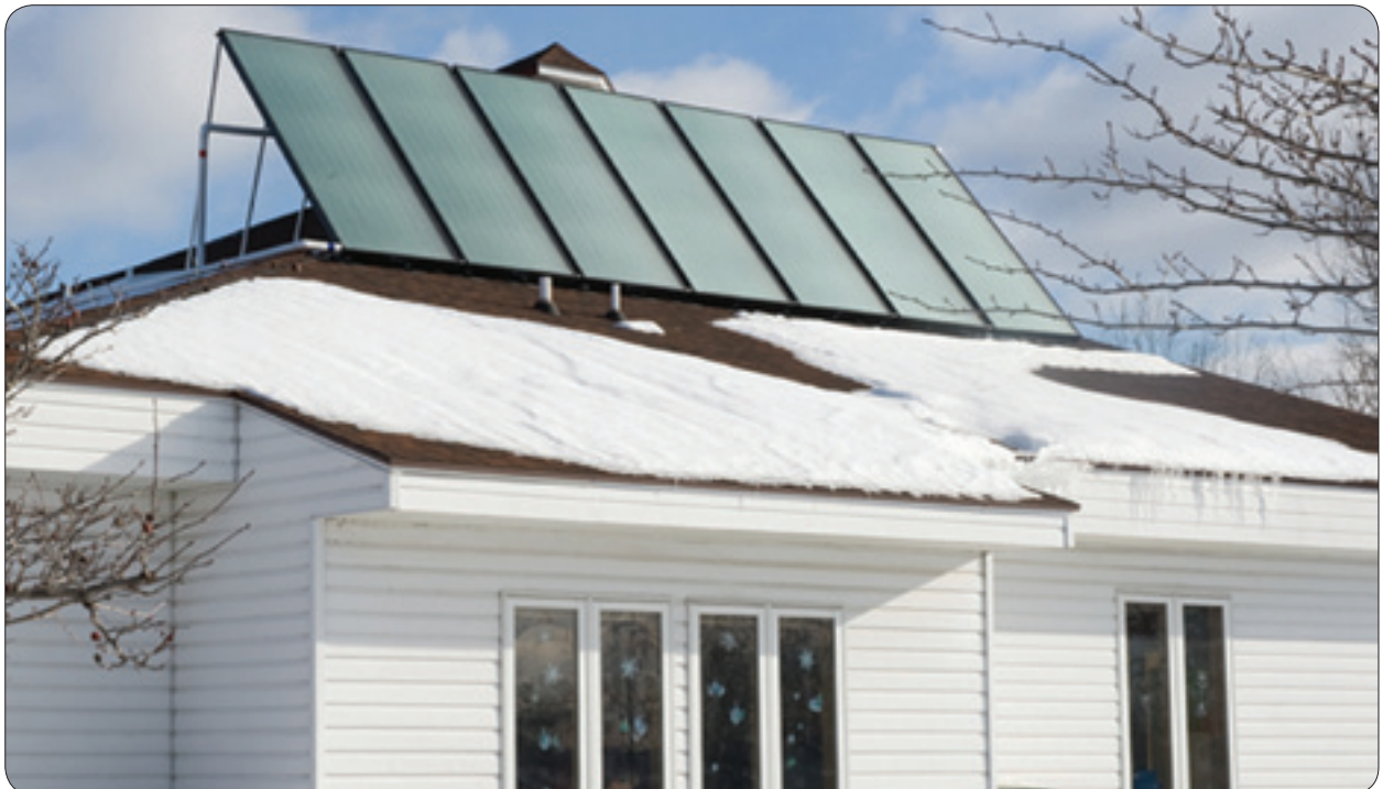
Gundersen Lutheran installed solar panels on the roof of its Child Care Center as part of a solar hot water heater project.
